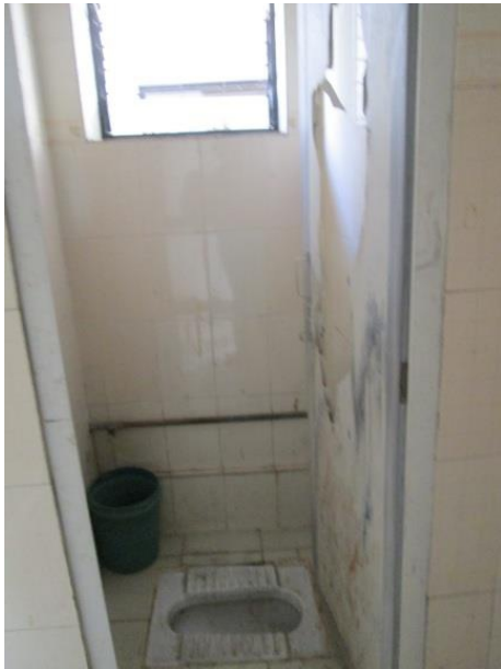
Fixtures not placed at child-accessible heights
