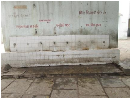
Fixtures not placed at child-accessible heights
