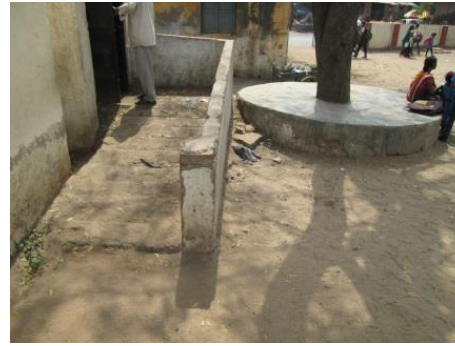
No compliance with CWSN standards
