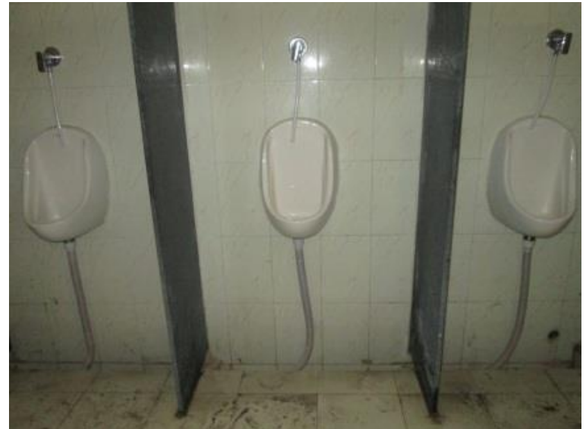
Inappropriate height and size of sanitation fixtures
